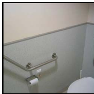
Figure 4: Example of wrong location fixing of grabrail which prevent optimal grip of grabrail
