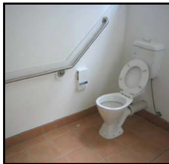
Figure 3: Example of grabrail fitted in the wrong angle but with correct location of fixing
